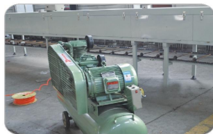
3. The first time drying section
