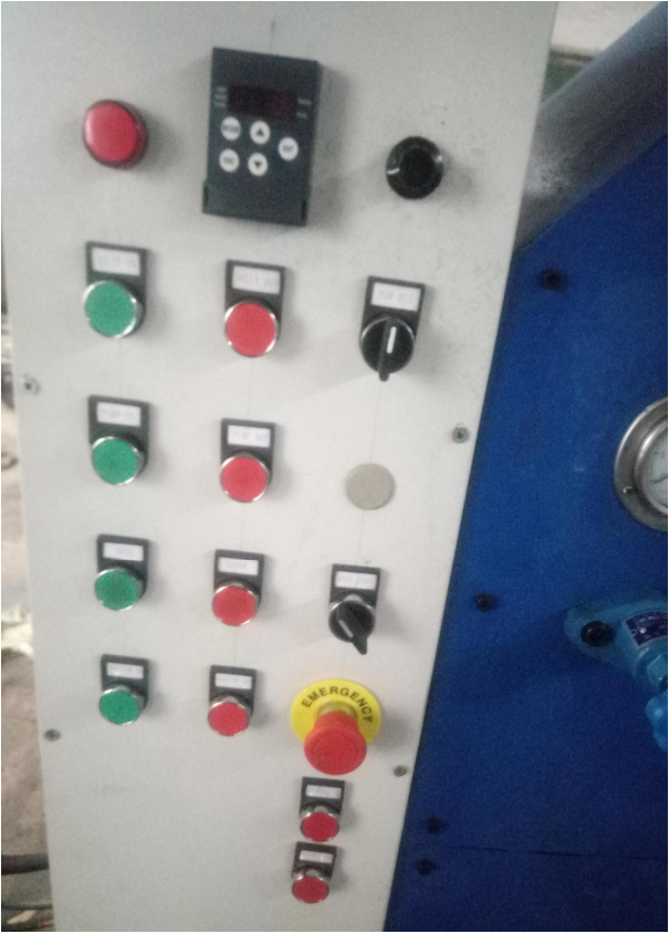
Electric control panel
