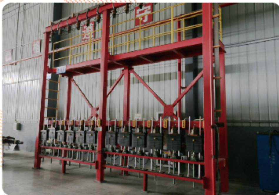
Electricity straightening equipment
