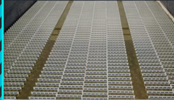
New aeration & oxygenation system
