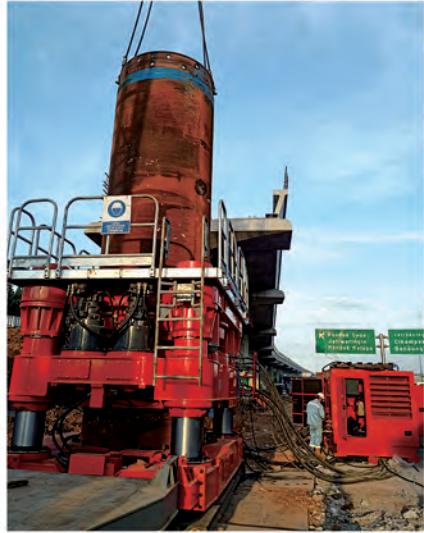
印尼雅万高铁拔旧桩 Old pile removing in Jakarwan High Speed Railway in Indonesia
