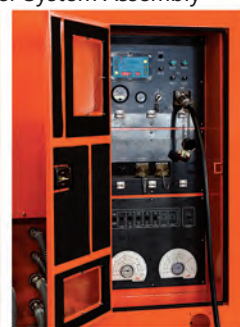
动力站电气系统 Power Station Electrical System
