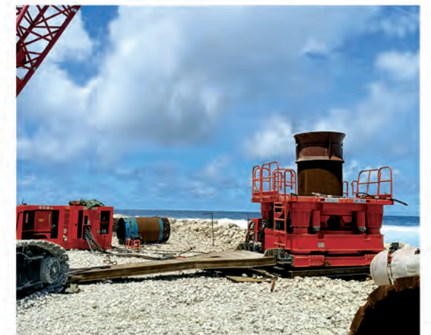
瑙鲁共和国码头桩基施工 Wharf pile foundation working in Republic of Nauru
