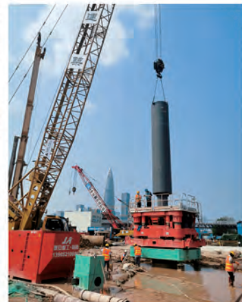
深圳湾插钢立柱施工 Insert the steel column working in Shenzhen Bay
