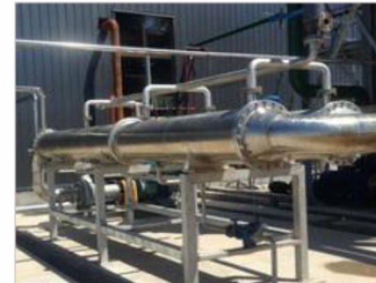
▲ Tubular Pre-heater 管式预热器
