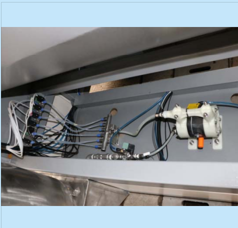
藥水加壓系統 Chemical pressurizing system
